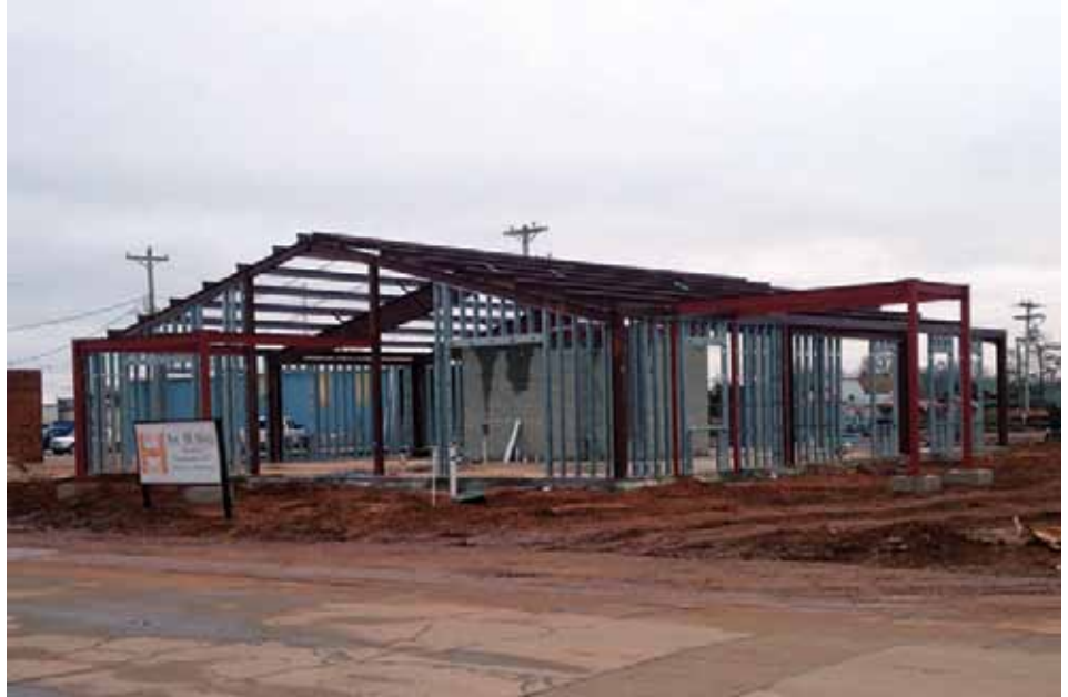
The new office facility in Buffalo is starting to take shape. Once the new building is completed, the old office will be torn down. NWEC is also expanding the existing warehouse to allow the large trucks easier access and to gain more storage capacity. Joe D. Hall Construction is overseeing the project.
